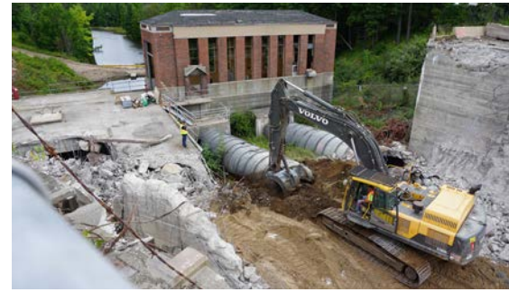
Excavator exposing the Boardman Dam penstocks during demolition (2017). Below, Sabin Pond and the dam after dewatering with the exposed stumps of trees cut during the dam's construction (2018).
