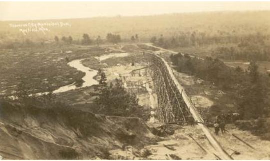
Construction of the Brown Bridge Dam circa 1920 (courtesy of Traverse Area Historical Society).
